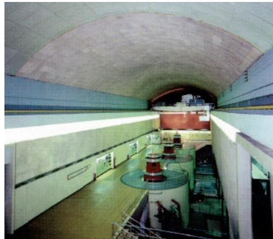
HPP Senj - underground facility
